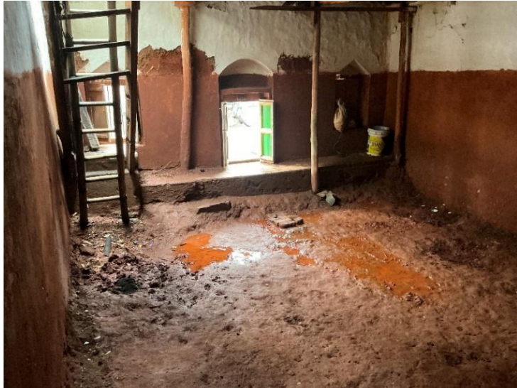
Figure 11: Water-clogged Matti due to Heavy rain at a Garadi Mane
