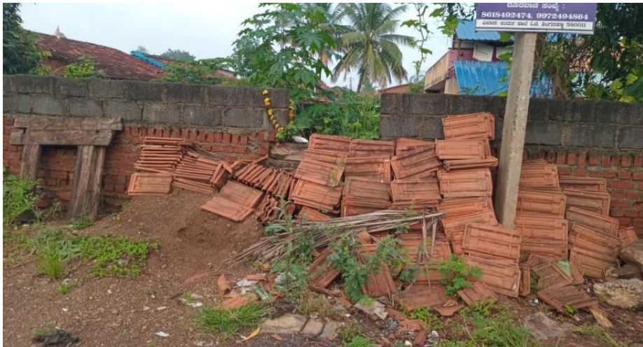
Figure 12: Completely devastated Garadi Mane at a village due to a lack of maintenance
